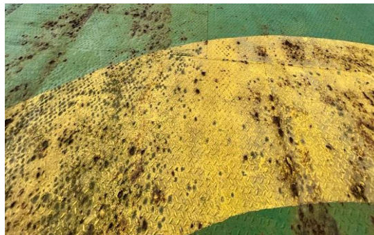
Fig. 5. Degradation of helideck surface around the Touchdown and position marking circle leading to reduced surface friction
