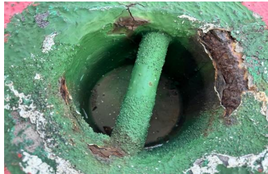
Fig. 4. Helideck surface degradation around the tie-down points
