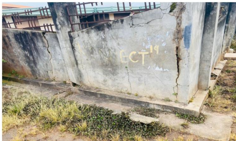
Plate 8. Buildings with cracks
