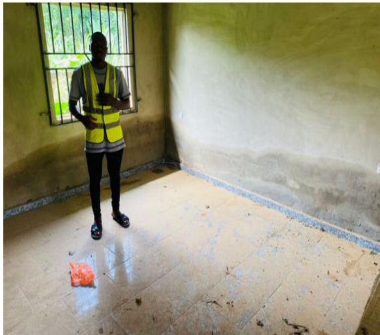
Plate 6. A building with damp, which leads to functional failures
