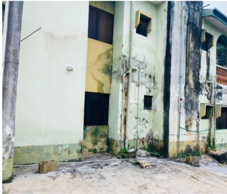
Plate 1. Buildings with functional failure as a result of damp
