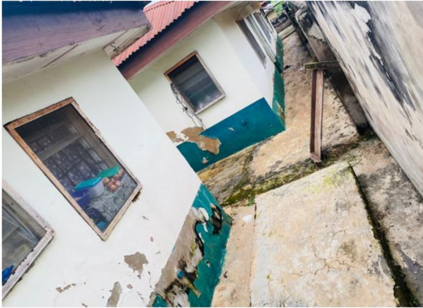
Plate 3. Damp in building which results in functional failures
