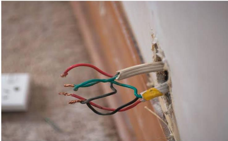
Plate 5. A building with electrical wiring defects which leads to functional failure
