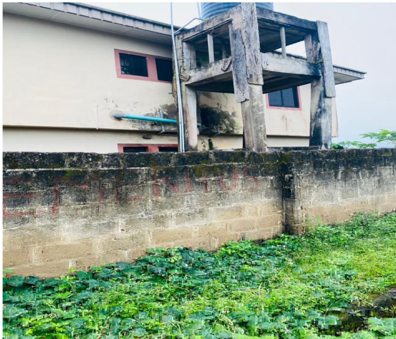
Plate 9. Buildings with plumbing defect
